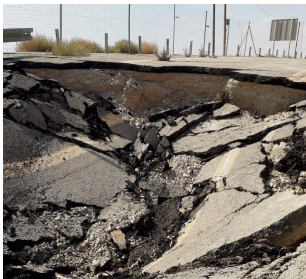
Fig. 6 – Collapsed road section in one of the sinkholes, Ein-Gedi.
