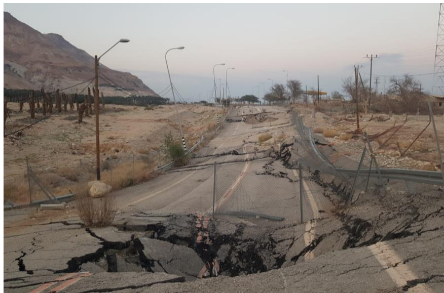
Fig. 5 – A section of the Jerusalem-Eilat road near Ein-Gedi (Dead Sea shoreline), that was recently abandoned due to opening of sinkholes.
